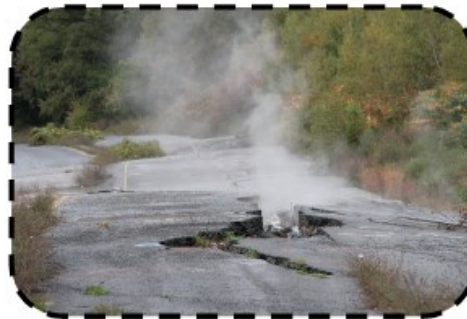
Smoke from the fire rises from cracks in the middle of a road in Centralia
